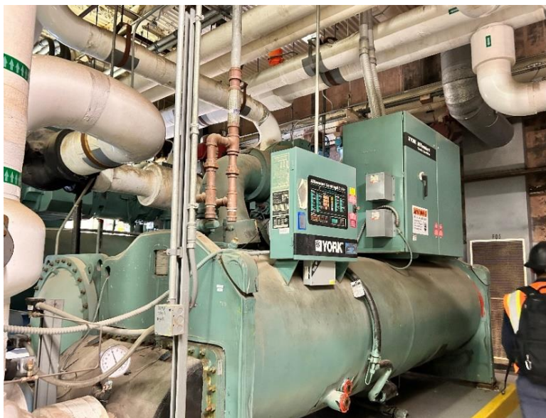
Chiller to be Replaced
